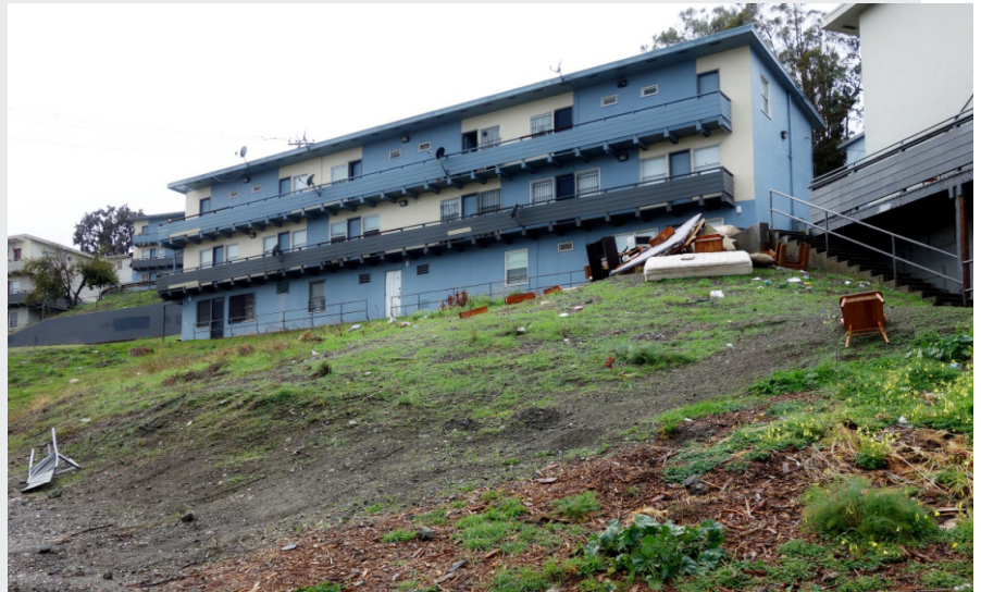
Potrero Terrace was built as temporary housing for shipyard workers during WWII. Seventy years later they are showing their age.
